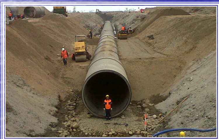
Sewage outfall of La Taboada (Lima, Peru). I.D.= 3.000 mm
