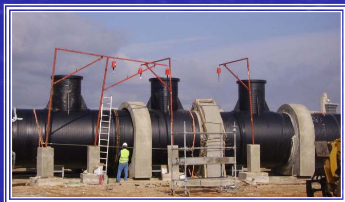
Algeciras (Spain) Power Plant cooling circuit. View of the diffuser I.D.=2.400 mm
