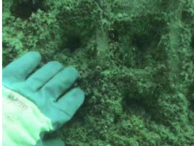
Figure 8: Deposits in windows of a tower
