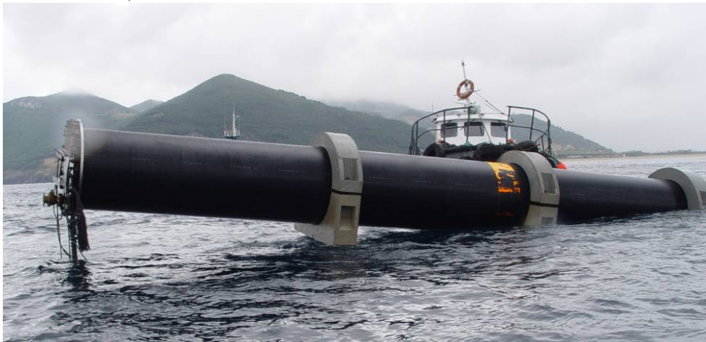
Figure 2: Sewage outfall of Berria (Spain). Solid wall pipe of 1600 mm.
