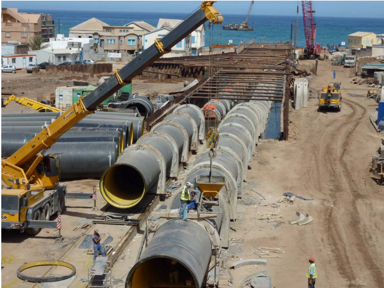
Figure 1: Desalination plant of Beni Saf (Algeria). Helioidally welded pipes of 2400 mm, produced by PPA&KRAH
