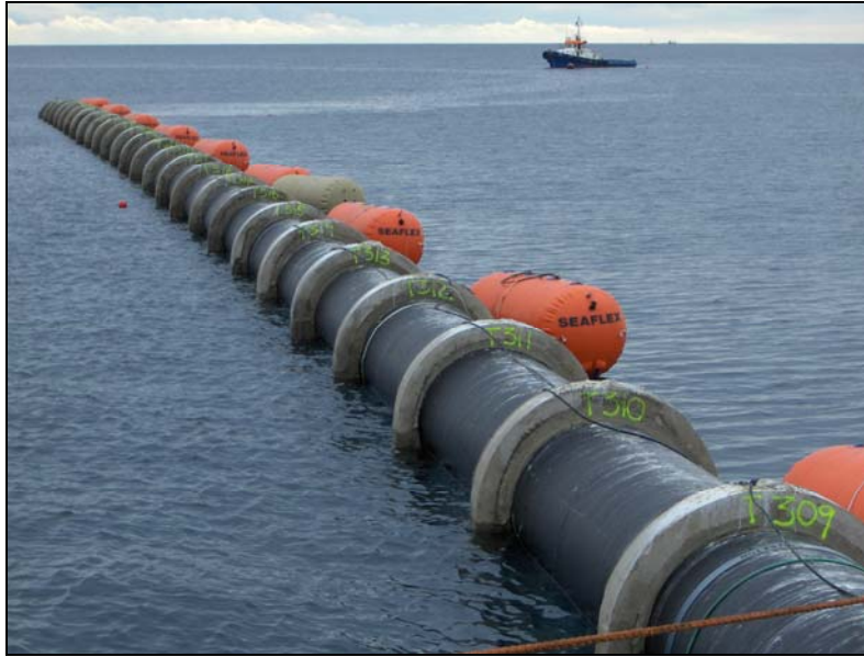
Figure 7 : Valdelentisco intake pipe, floating before submersion
