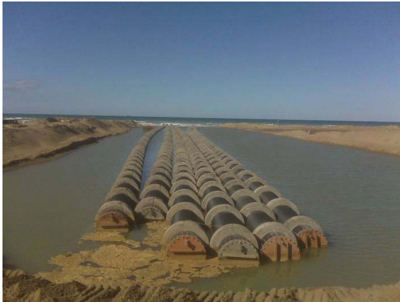
Figure 9 Mostaganem: pipes floating in a trench excavated at the beach, before transport and sinking
