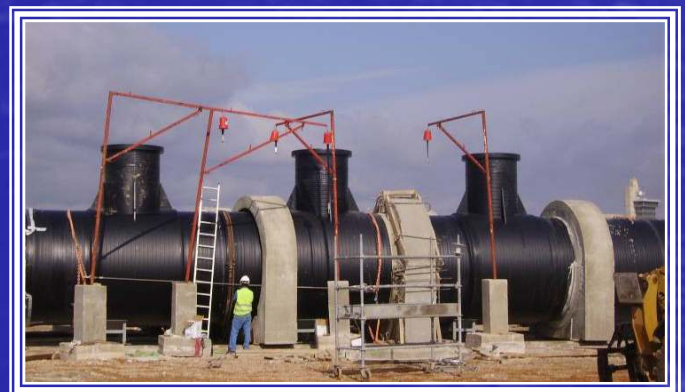
Algeciras (Spain) Power Plant cooling circuit. View of the diffuser I.D.=2.400 mm
